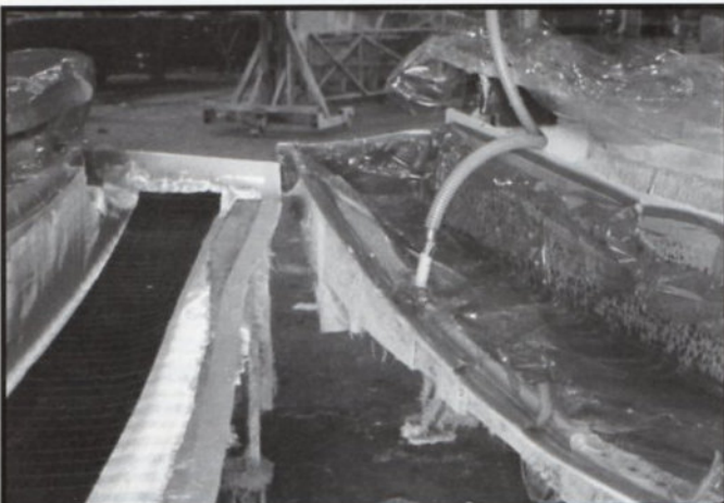
Beam tops are shown here, one having the first of many layers of Carbon fiber pre-fitted, while the other is being vacuum bagged. Excess resin, extracted by the vacupressure system can be seen in the white bleeder material
